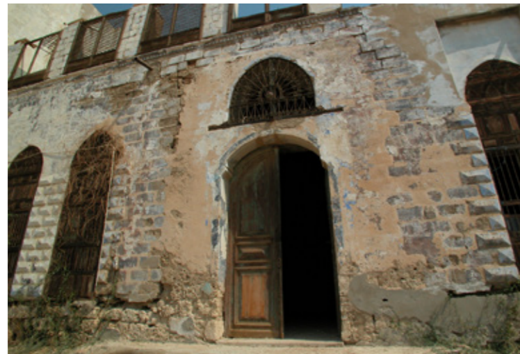
Attached pictures show the architectural study of the facades of the western building. The main feature of this façade is engraving, arches, doors and semi-circular windows
