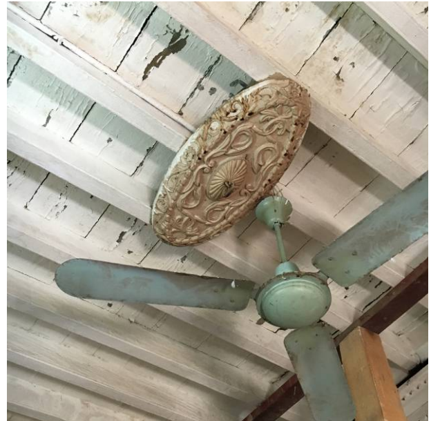
Ceiling decorative element, to clean, restore and put back in place.
