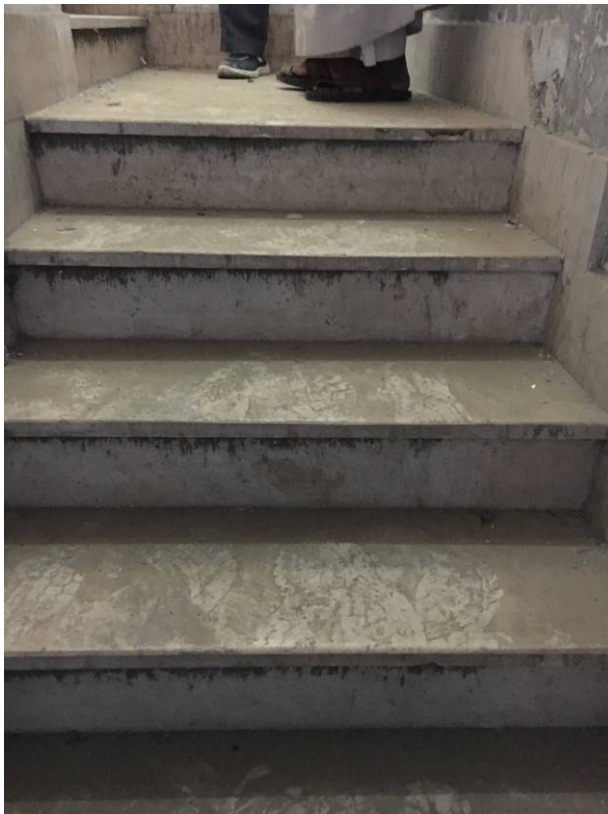
New staircase, to be cleaned and arranged ; no need for replacement, unless there is a will to put back into shape the original type of stairs (stone and mortar, with wooden edges)...
